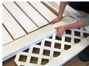
Step 2: Put C-Channel on both sides of lattice and place in mid-rail.
